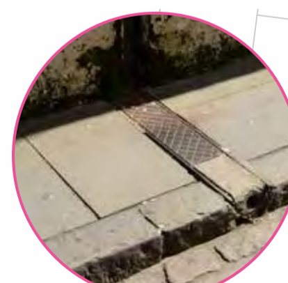
Decorative iron surface drainage channels
