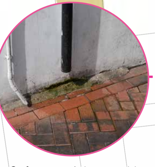
Surface water drainage provision is variable throughout street Inadequate drainage gullies and down pipes discharging onto road surface with no channelling or low spot - some in areas of café seating
